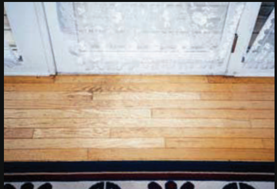
Dirty floors with finish totally worn off.
